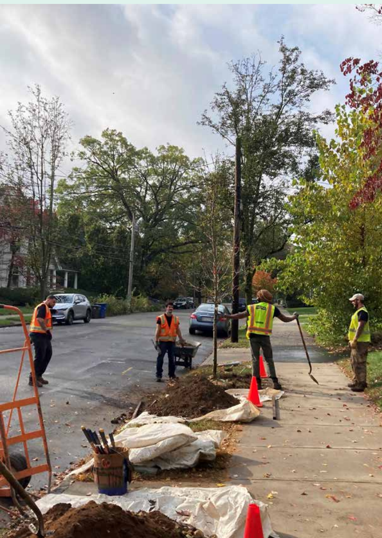
Greenskills crew members straighten street tree during planting. Courtesy photo by URI.
